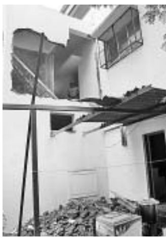
A file photo of the illegal construction.
